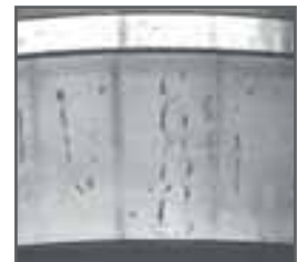
Rust and Corrosion
